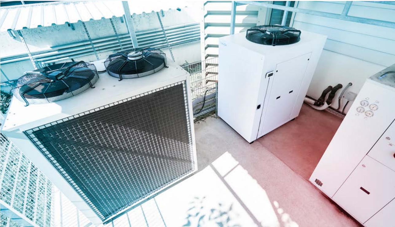
Sufficient cooling capacity even at an outdoor temperature of more than 45 °C
