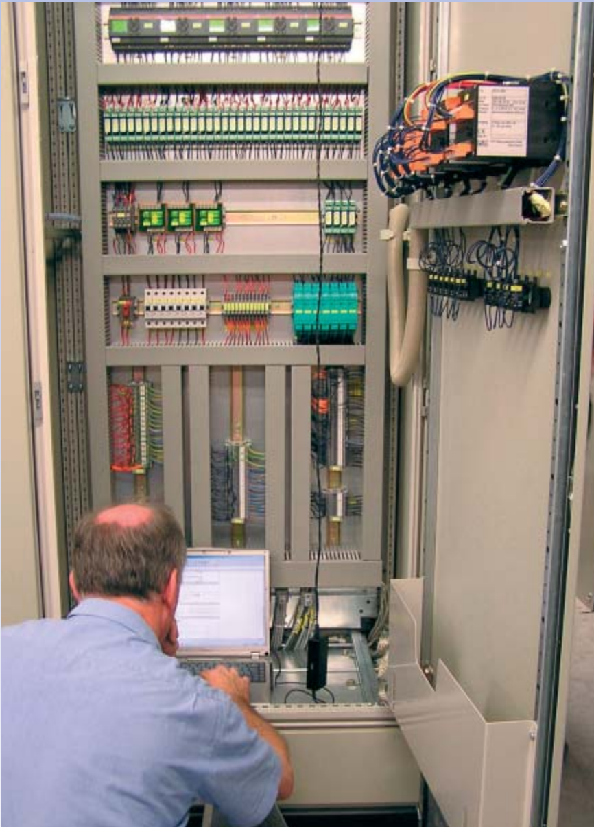
Fieldwork: The LAUDA service technician checks the electric connections of the systems.
